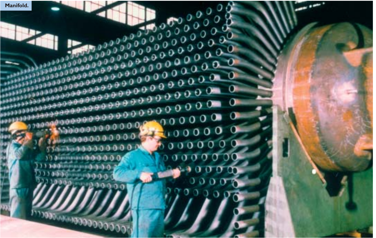
Tube to manifold joint welds of a waste heat recovery boiler.
